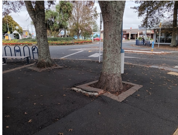
FIG. 4-1: Broken pavement due to tree roots pushing up.
